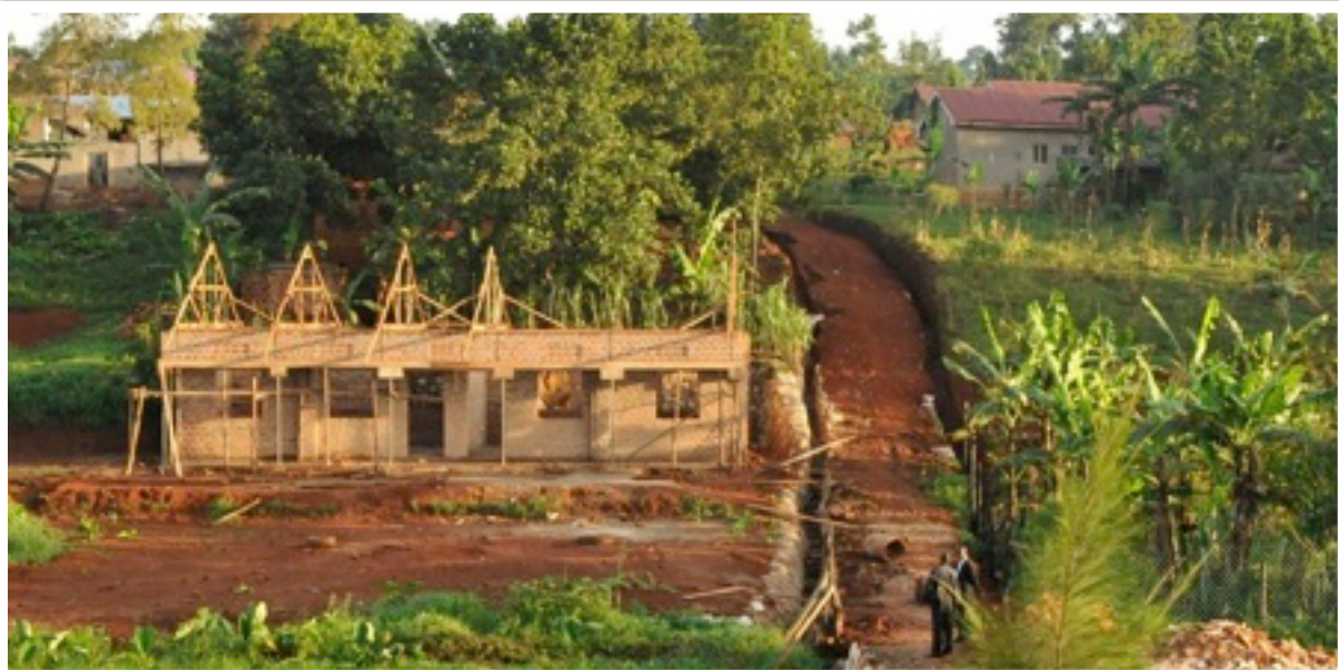
Looking across the valley, the low evening sun illuminates the construction of a new classroom block.
